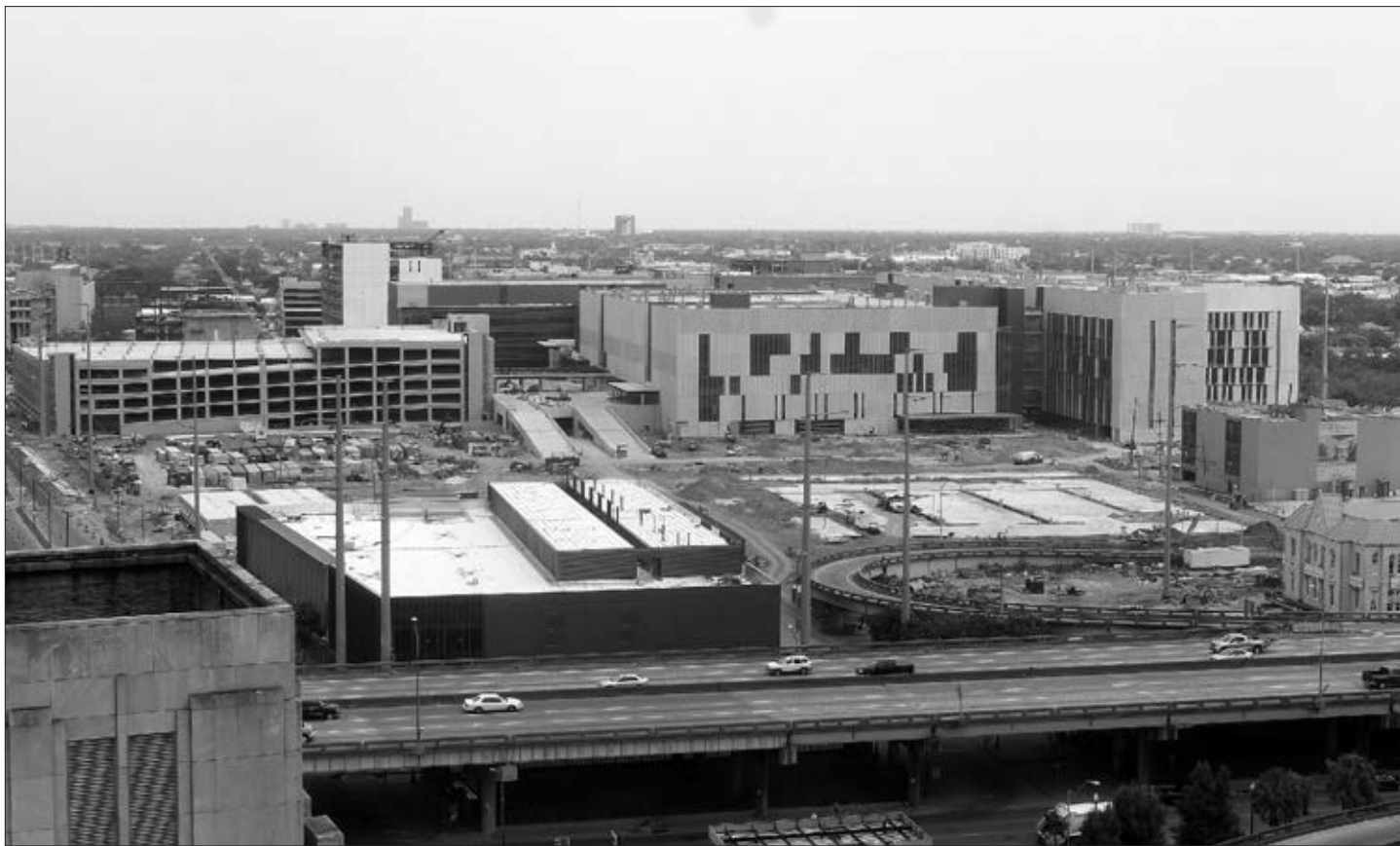
Construction site with Claiborne Avenue Overpass in the foreground. For more details, visit http://www.newhospital.org/ .
